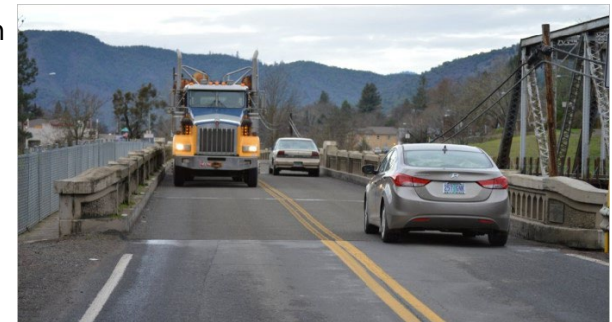
The narrow bridge is frequently struck by passing cars
